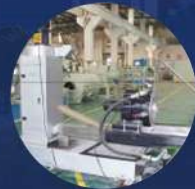
Dewatering Drying Pellete Storage System
