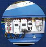
The motor overload protection function is automatically stopped after overload
